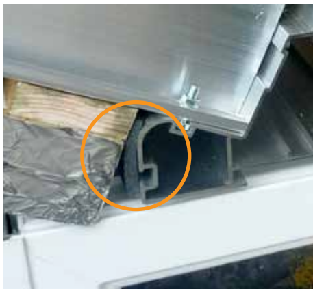
22. Apply 60mm foam to up stand of ring beam prior to installing plasterboards as shown.
