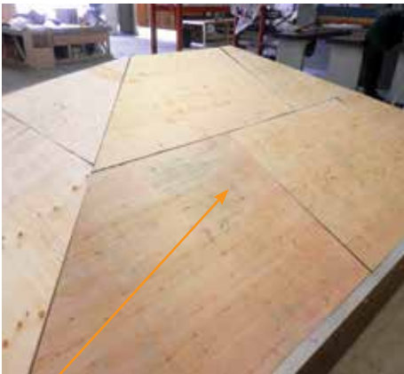
16. Cover the entire roof with 12mm plywood, fixing at the same time with either nails or screws onto hips & rafters using a minimum 35mm nail or screw (not supplied).
