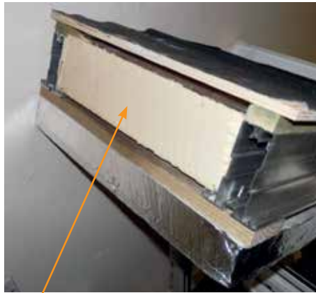
14. Once all of the frame work of the roof is assembled, start work fitting 100mm insulation between rafter & hip. These are all numbered, for example:- S1 / S2 / S3 / S4 / S5.
