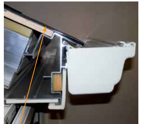
18. Once the plywood is fitted, cover the roof with breathing felt. Ensure at least 50mm of felt runs in to the gutter, this can be trimmed back later.
